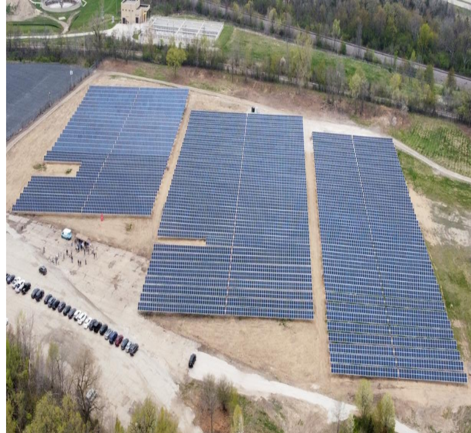
Fox Metro Water Reclamation District Annual Production = 3.3 million kWh/year Lifetime Production = 82.5 million kwh's
