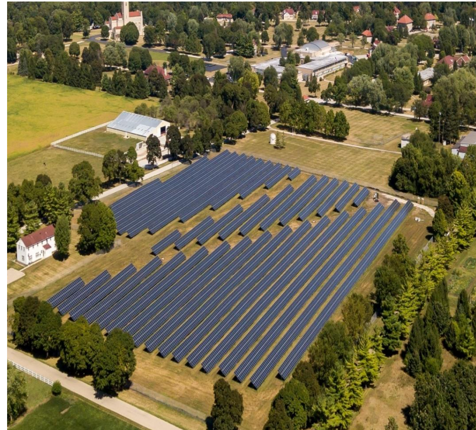
Mooseheart Child City & School Annual Production = 3.5 million kWh/year Lifetime Production = 84.5 million kWh's
