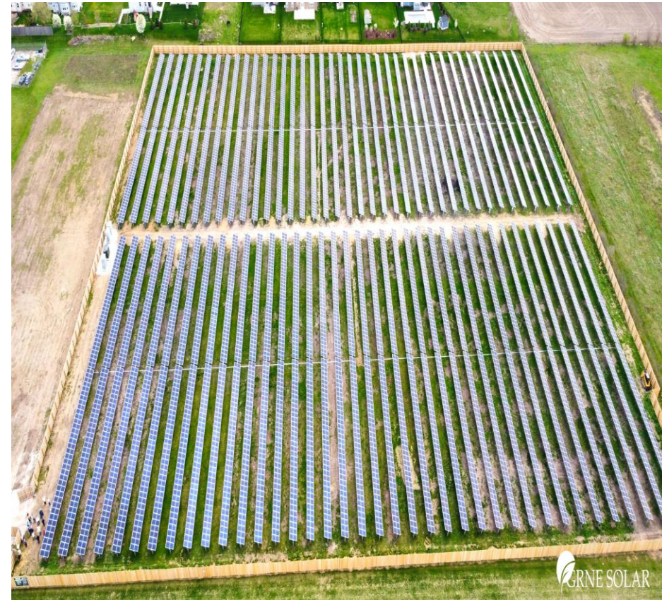
Kendall County, IL (Public Safety Building, Courthouse and Health Services) Annual Production = 3.3 million kWh/year Lifetime Production = 82.5 million kWh's
