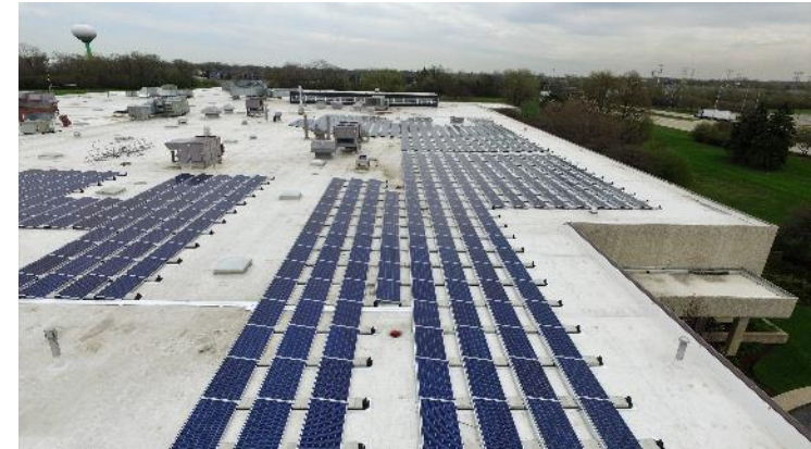
Spraying Systems Glendale Heights, Illinois System Size - 433.50 kW 1,333 modules
