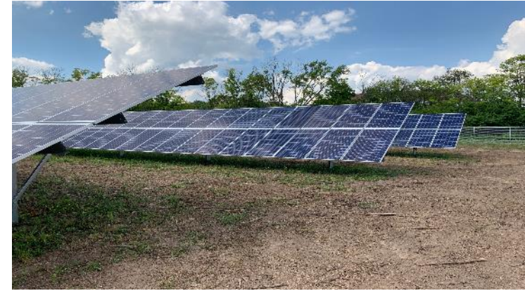
Duke Energy West Lafayette, IN System Size – 2.4 MW 7,000 modules
